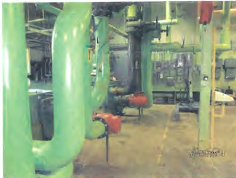
South Boiler Room – Power Panels
