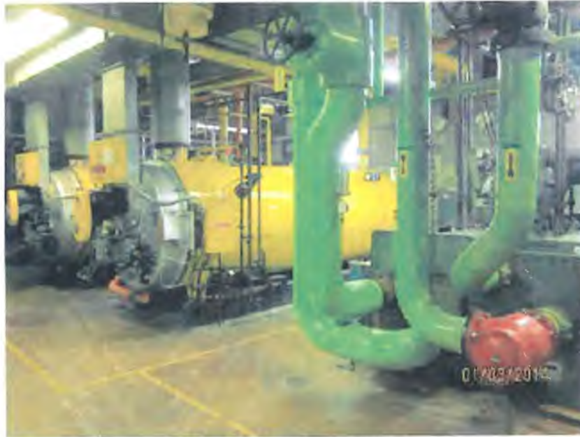
South Boiler Room - Boilers
