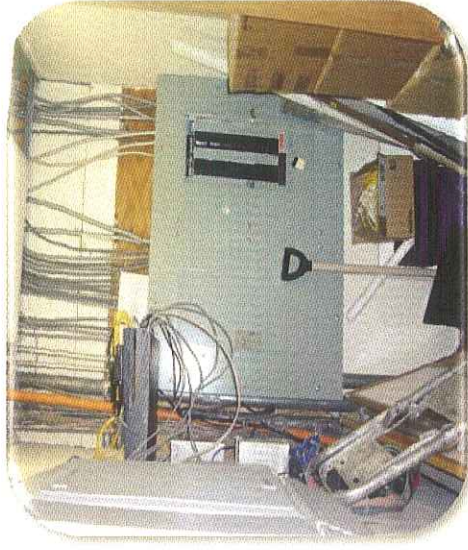
Photo 3. Mostly two panelboards were observed in each tenant closet. Closets are, however being used as a storage in violation of National Electrical Code.
