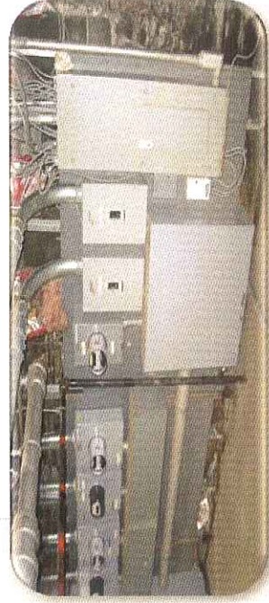
Photo 2 Housekeeping Panelboards and Tenant/Housekeeping Meters Located in the Basement.
