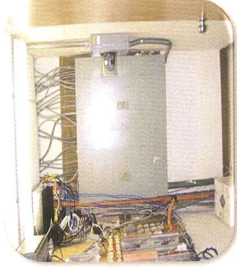
Photo 2 Double Tub Electric Panelboards Provided in the Electrical Closet in Each Tenant Space. However, in Violation N.E.C code, Closets are Also Being Used as Storage Space.
