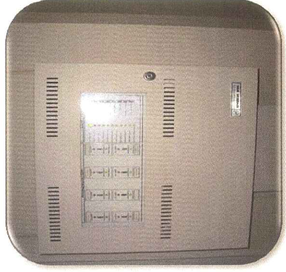
Photo 4 Main 8-Zone Fire Alarm Panel Located in the Main Lobby at Ground Floor.
